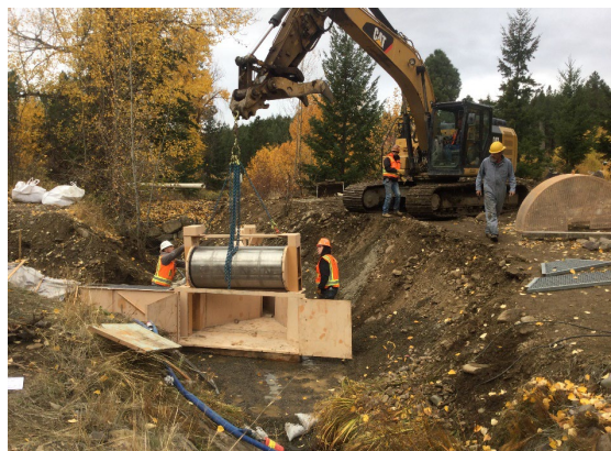
Figure 14. Fish screen installation on Swauk Creek to accommodate the two diversions that were consolidated. WDFW Yakima Screen Shop provided the screen.
