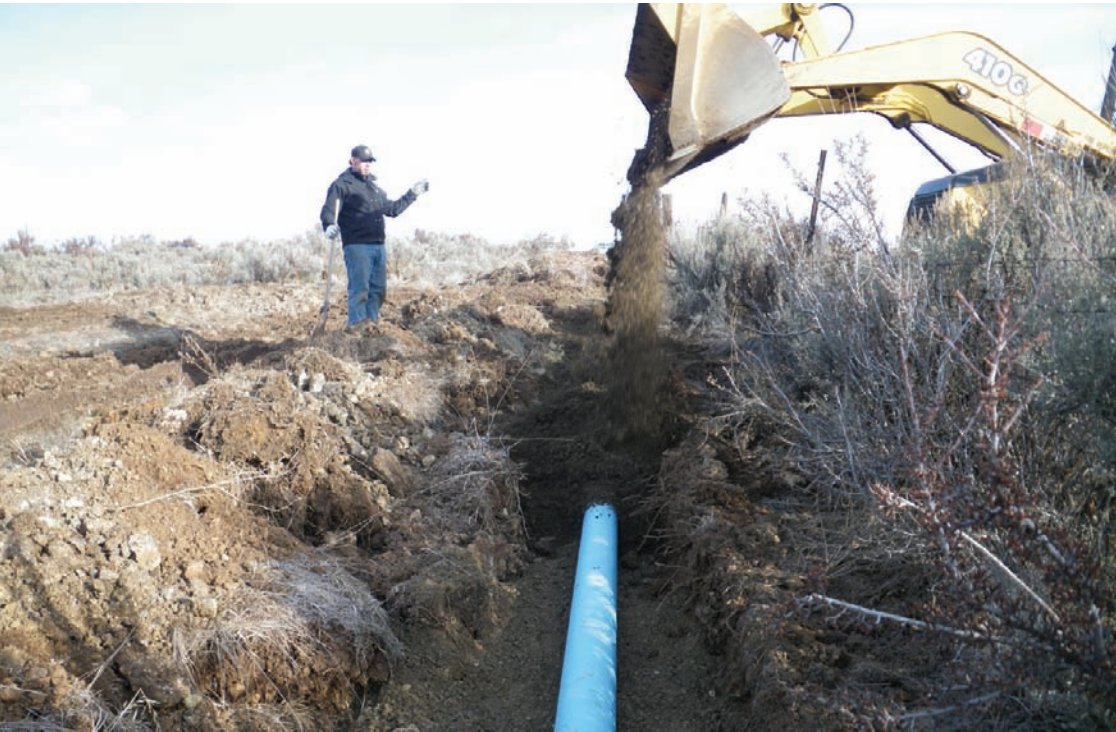
A landowner used funding from the Small Cost Share Program to help install pipe to deliver KRD water.
