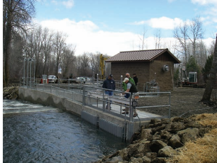
The new Keach/Jensen diversion facility, part of our long running Manastash Creek Restoration Project.
